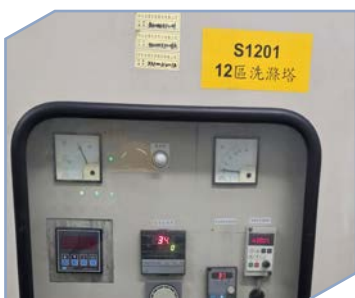
Area 12 S1201-502 Scrubber 30HP Exhaust Fan
