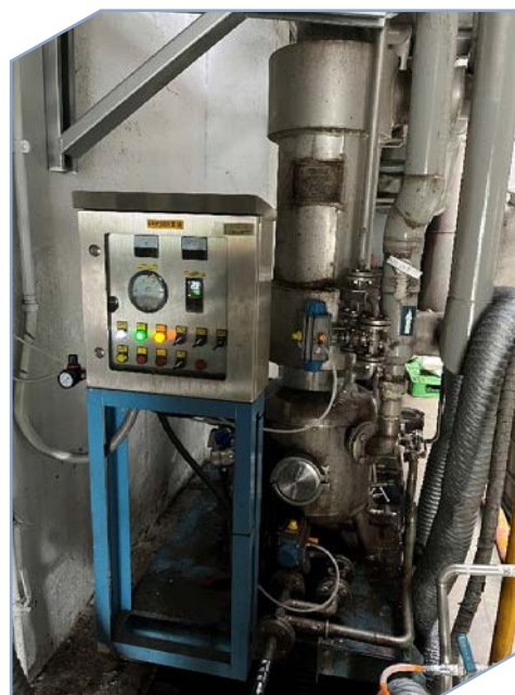
Vacuum pump and water recovery system
